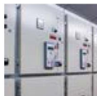
Electrical switching rooms
