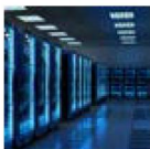
IT and server rooms
