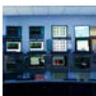
Control rooms, technical rooms
