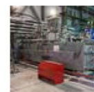
Closed transformers, generators
