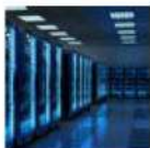
IT and server rooms
