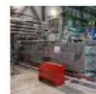
Closed transformers, generators
