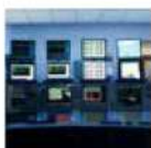
Control rooms, technical rooms
