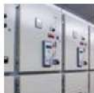
Electrical switching rooms
